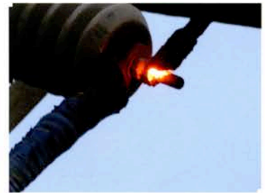
Overheating Cable riser
