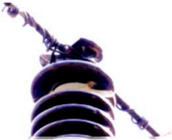
Crack and erosion Post insulator / conductor
